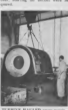
TURBINE HAULED away required torch cutting of ducts which were imbedded in concrete. ORA TURBINA tabata liki, mester a usa coriamento cu torch pa saka e tubonan hancho for di concrete.
